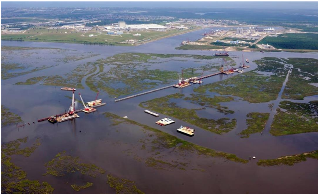
Construction of the IHNC–Lake Borgne Surge Barrier. Source: Southeast Flood Protection Authority–East.
